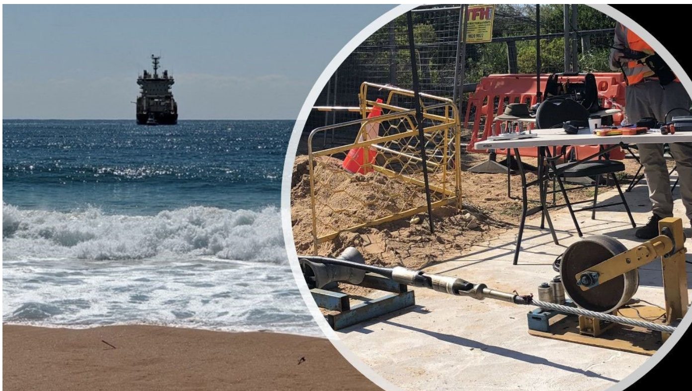
JGA South Cable Landing in Sydney, Australia
